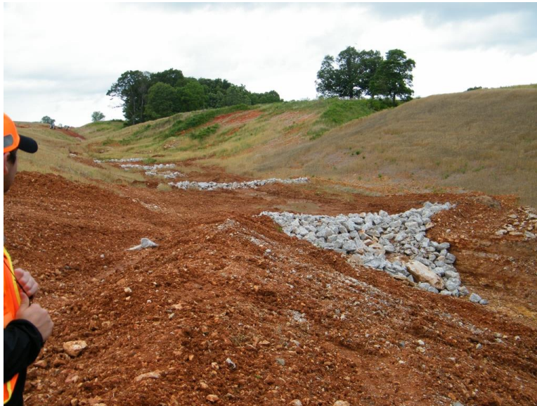
Figure 3.2: Photograph of the site chosen for the first field test. One inflow stream was from the left side of the photo, which enters the small and shallow basin. A second inflow stream is pictured in the background, which included a series of small basins with intermittent rock checks. Photo taken by Bryan Signorelli (AHTD) on June 18, 2015.
